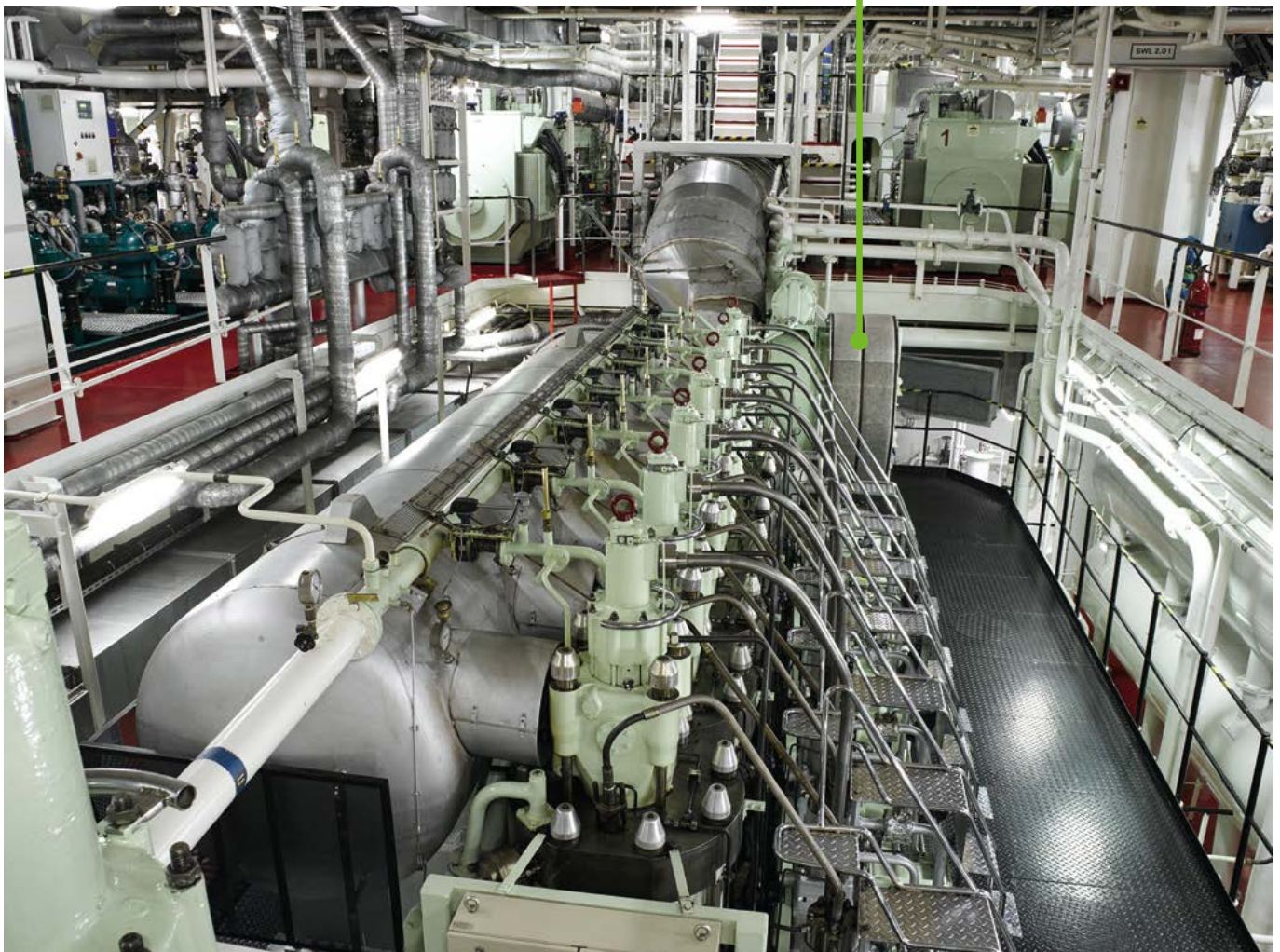
Air intake ship engine
