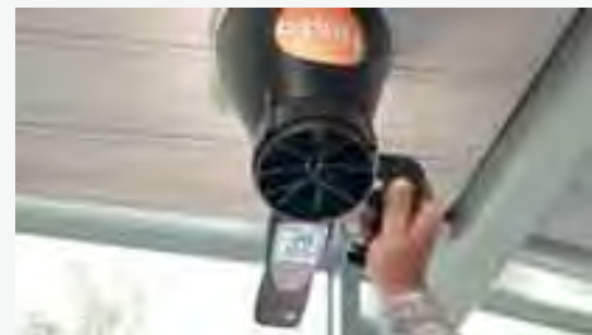
Monitoring ingoing air in a disc outlet
